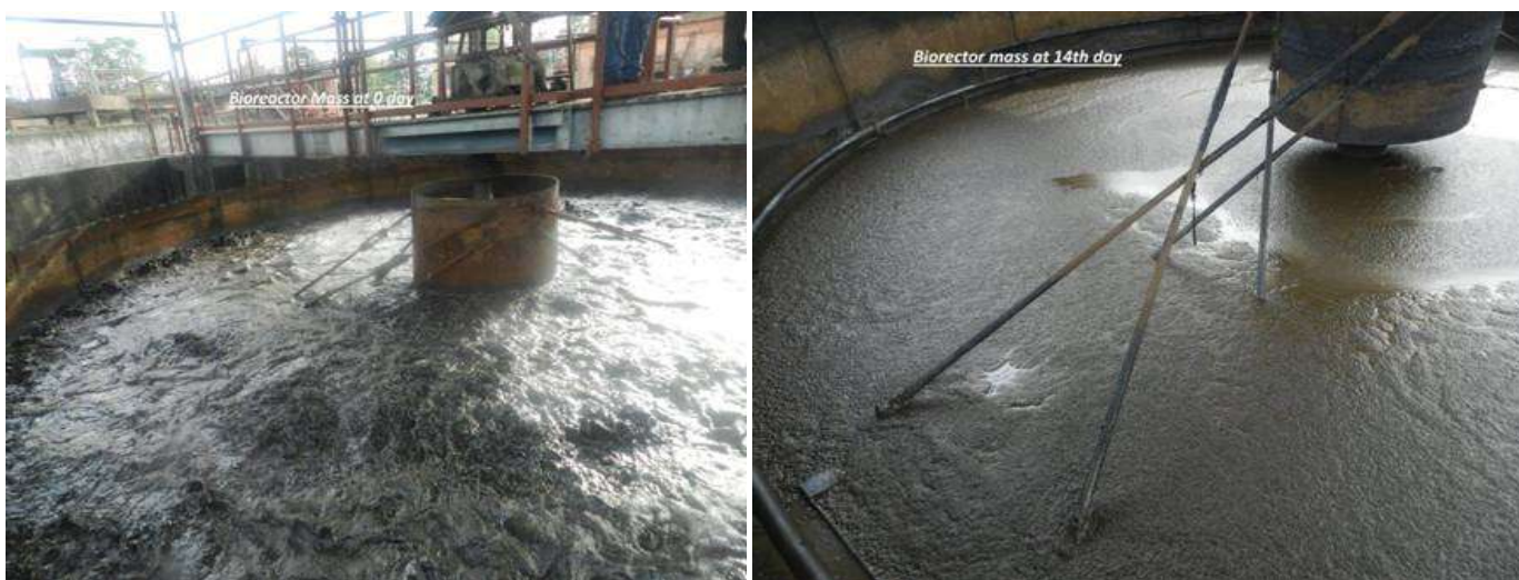
Bio-remediation facility of BGR
